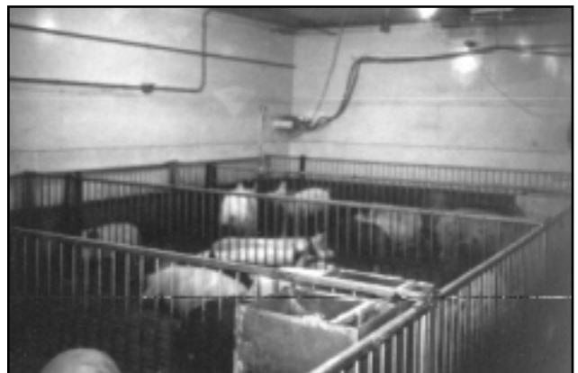
Figure 4. In-barn sensor installation setup
