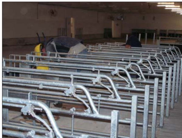
Construction crews are busy installing walk-in, lock-in stalls in the gestation room
