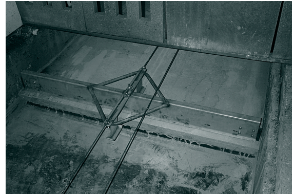
Figure 1. Scraper blade that was pulled over the false flooring. The manure pit has two drains, one at each end, through which the scraped manure was drained to the sewer line.
