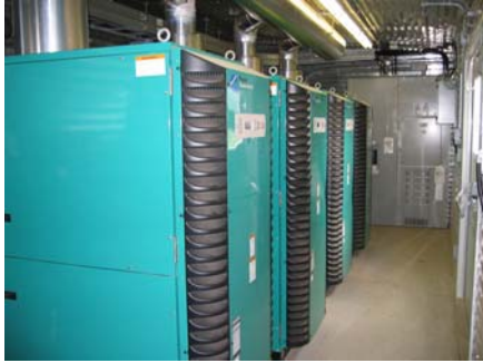
Four Capstone micro-turbine engines operating on methane produced from liquid hog manure in Saskatchewan. Turning methane into electrical energy will likely be a practice capable of netting carbon credits.
