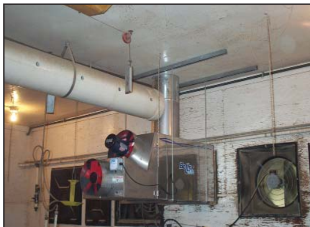
Figure 1. Heat exchanger installed in a grow-finish room.
