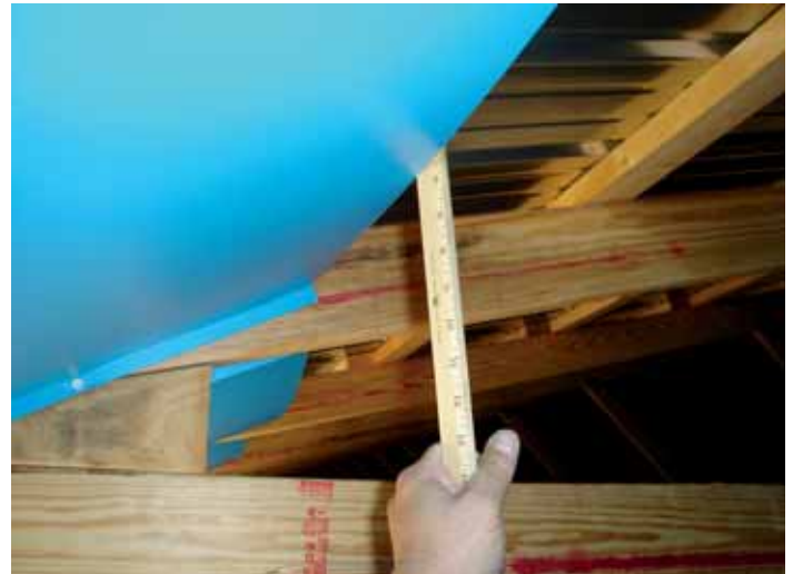
Figure 5: Incorrectly installed insulation stops that result in restrictions to air flow to ceiling inlets. While the upper rafter chord is a 2"x6", the actual inlet width when accounting for the purlins is only 4 inches. At this site, a minimum of 6" was necessary to meet the ceiling inlet capacity as installed.
