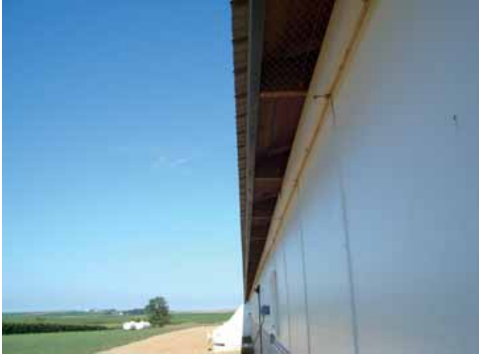
Figure 4: A correctly constructed eave inlet to an attic. Note the lip on the metal soffit material which acts as a deflector to minimize snow drift into the attic area
