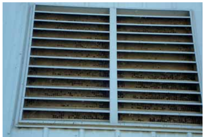
Figure 3: A gable end attic inlet obstructed with dirt and lint covering the screening material
