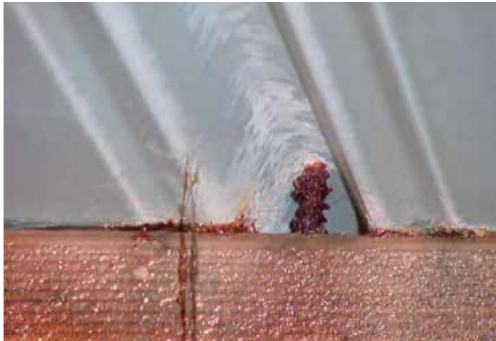
Deterioration of sheathing screw, sheathing and wood (Photo courtesy Yves Choiniere)
