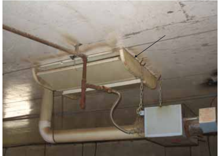
Leaks between the ceiling and inlet allow moisture into the attic
