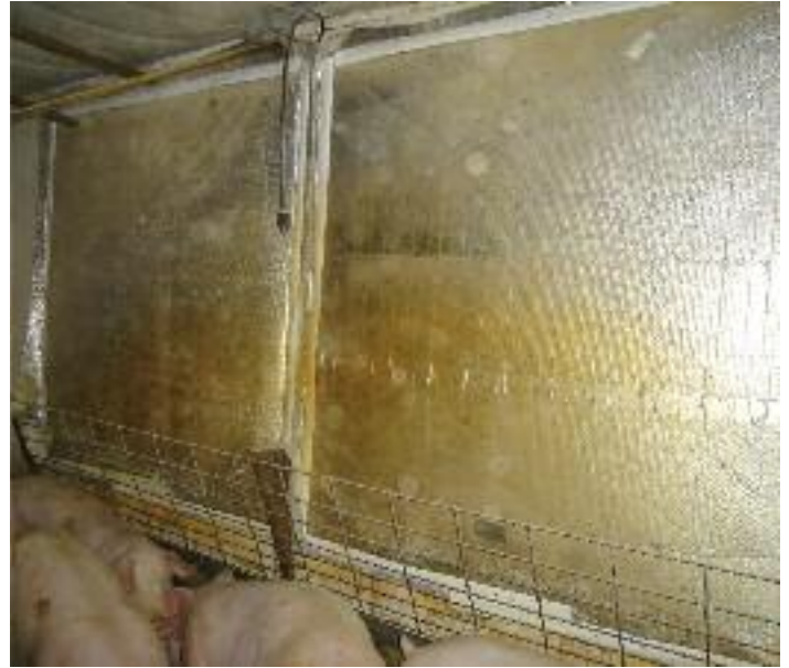
Figure 2: Insulated fans in a finishing facility
