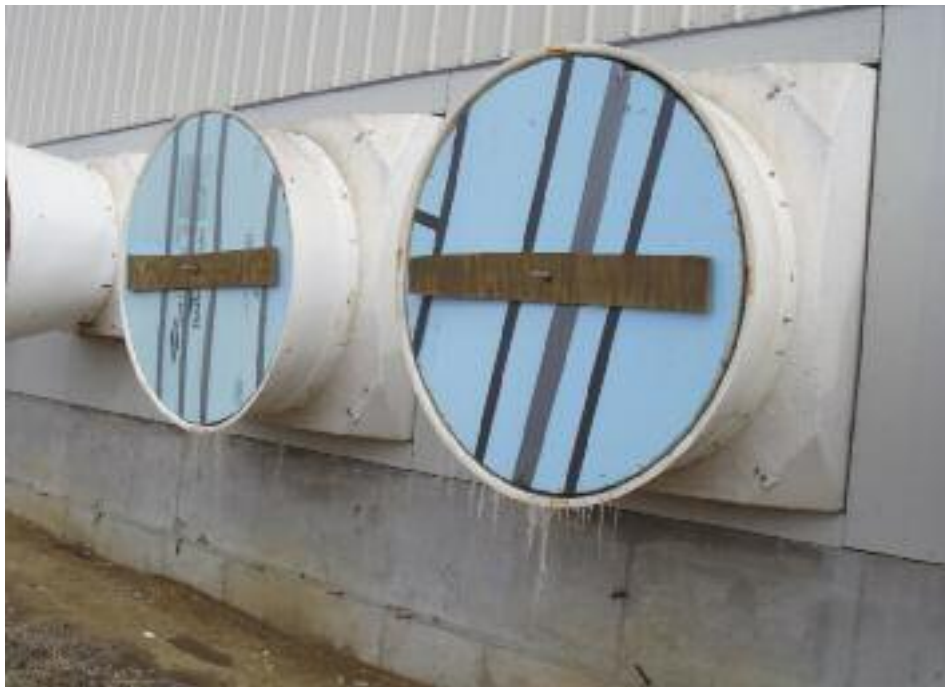
Figure 3: Insulated fans with cover on the cold side of the fan. Note the moisture condensation forming on the fan shrouds
