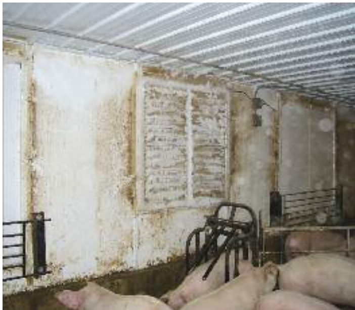
Figure 1: Insulated panels for winterizing unused fans. Note the ice on the uncovered fan shutter
