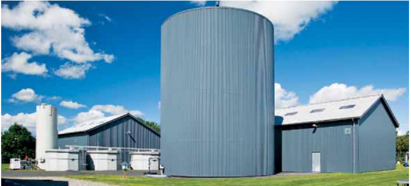
This bio-digester on a Danish farm produces methane, which is burned to provide electricity for the farm and also for sale into the grid
