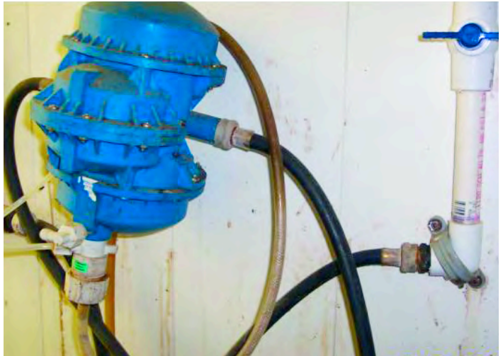
Water medicator rated at 26.5 litres (7 gal)/minute incorrectly connected to 19 mm (3/4") inside diameter piping with 13 mm (1/2") washing machine hose.
