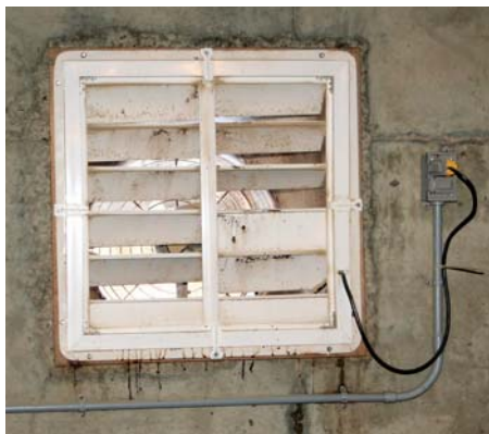
Over-ventilation is the most common reason for excessive energy costs, says the Prairie Swine Centre's Dr. Bernardo Predicala
