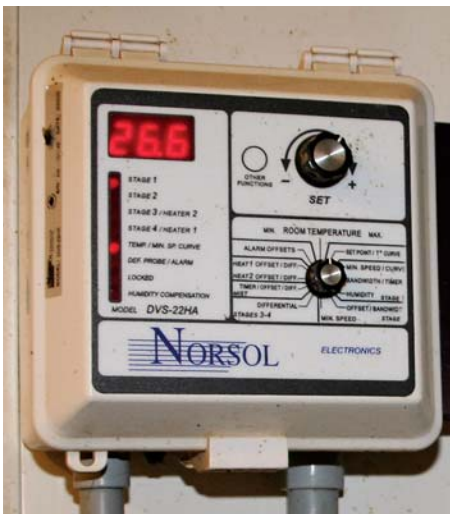
Modern ventilation controllers are very sophisticated, but can be intimidating
