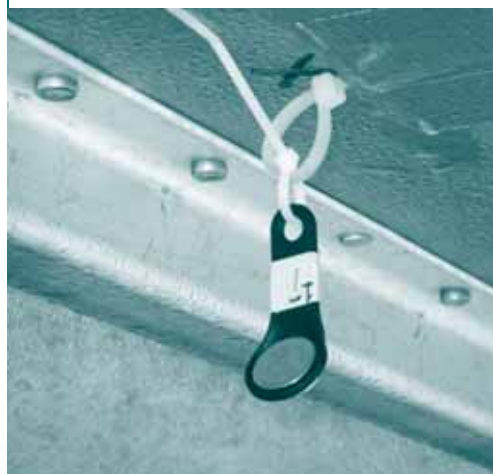
Temperature and humidity sensor attached to ceiling of a vehicle compartment.
