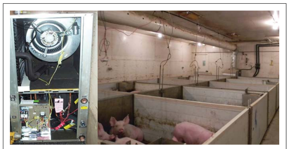
Figure 1. Heat pump used in the geothermal system installed in a grow-finish room.
