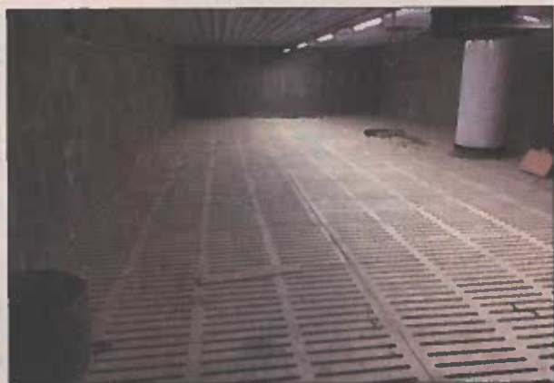
Slatted floor to edge. Solid areas can be easily made on the slats and removed if necessary at a later date.
