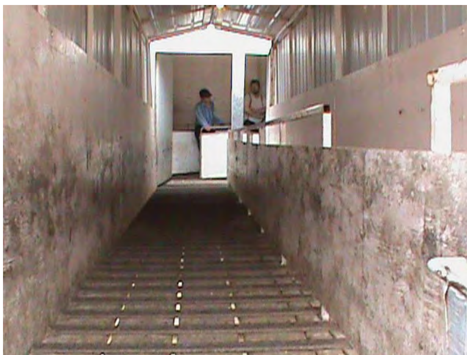
Figure 1. Covered hydraulic loading ramp with manway (looking down ramp from truck entry)
