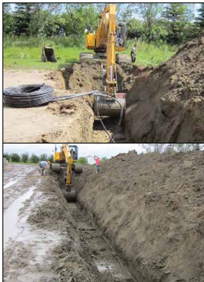
Building of a trench with a horizontal loop of polyethylene pipes as part of the Prairie Swine Centre geothermal system
