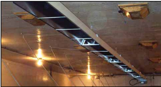
Infrared radiant tube heater
